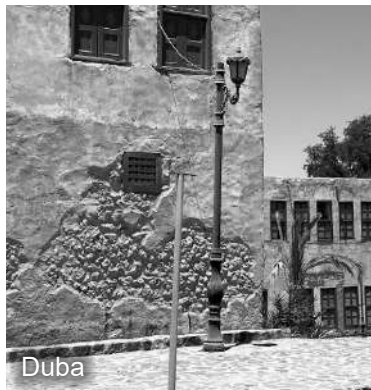
Dubai Erosion of plastered finish to base of wall
